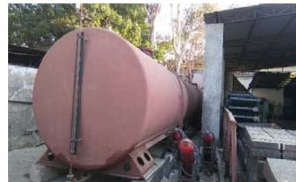
Oil Tank at our factory for making Oil cooled Transformers
