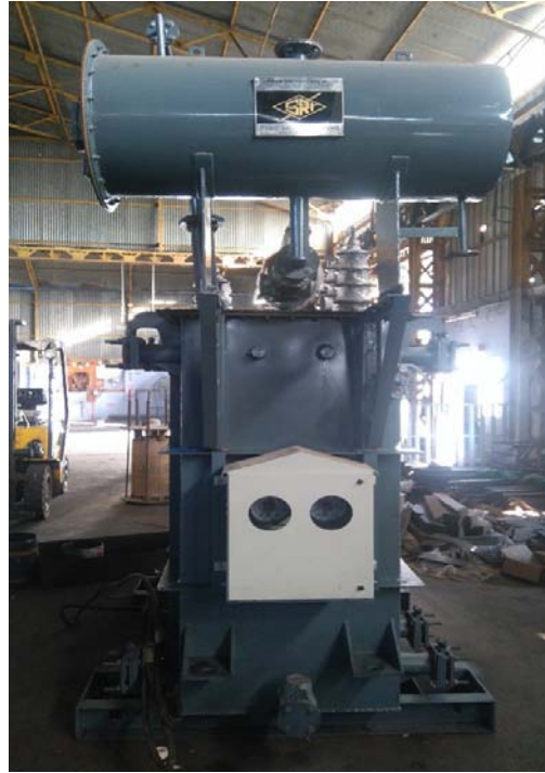
EHV Transformer of 5 mVA Capacity
