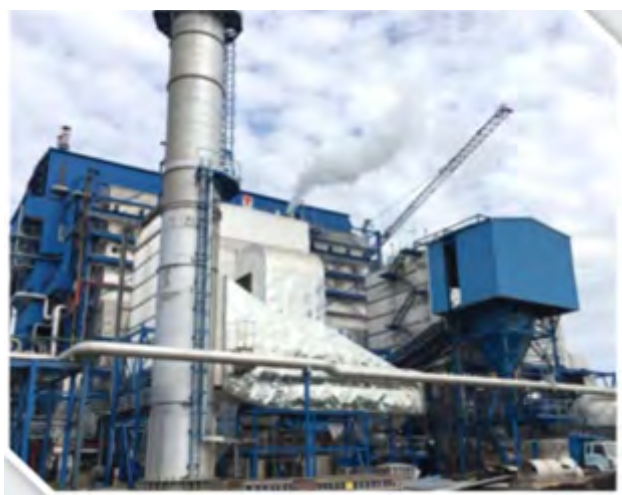
Thermax's largest boiler installation in Thailand.
